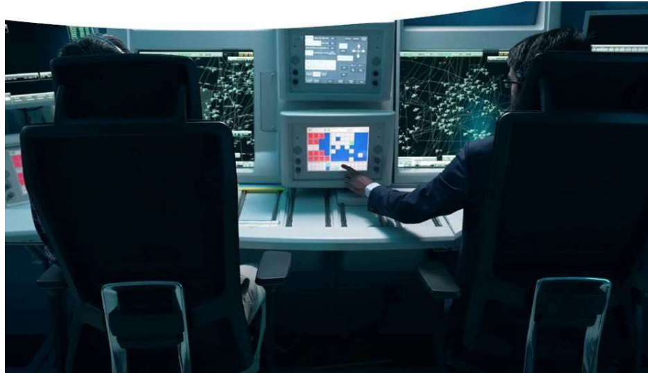
ENAIRE air traffic controllers at a control post with new voice communications
